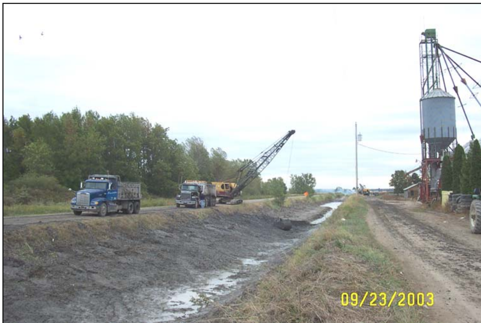
Excavated sediment and soils being trucked off-site during a drain reconstruction project.
